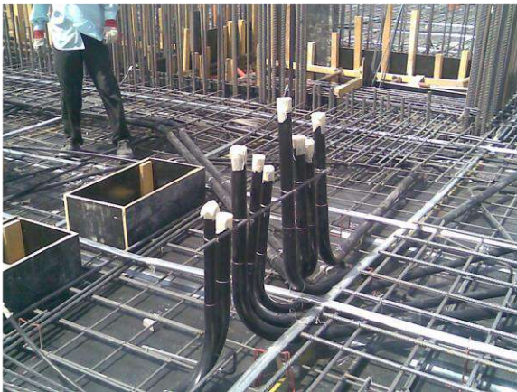
Electrical & Drainage services
