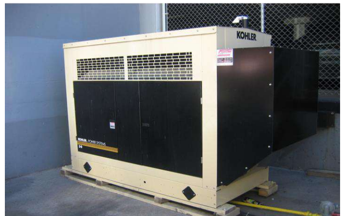
Supply of Generator
