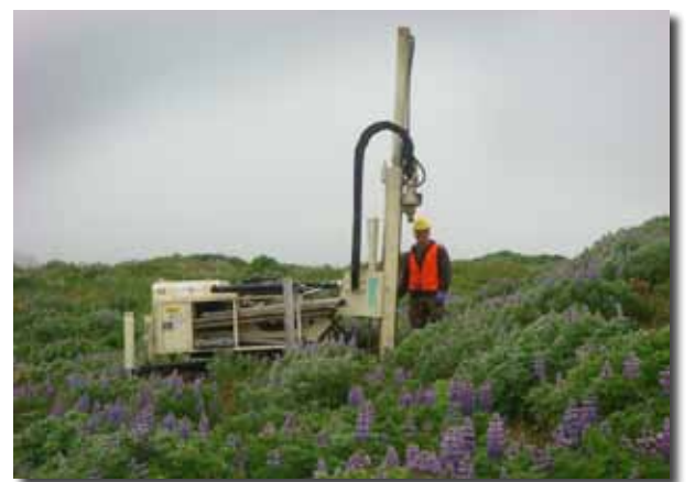
The relatively small size of the Geoprobe® 66DT makes it well suited to ship to remote areas of Alaska, such as Kotlik, Barrow, Quinhagak and Atmautluak. Here, soil samples are collected at this site on Shemya Island.
