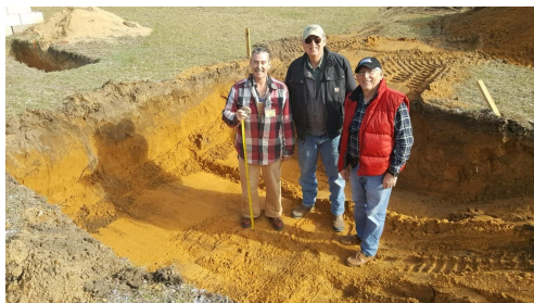
Kevin, Steve and Dennis stand in the foundation hole of the trap house.
