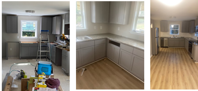
Cabinets, Countertops & Appliances
