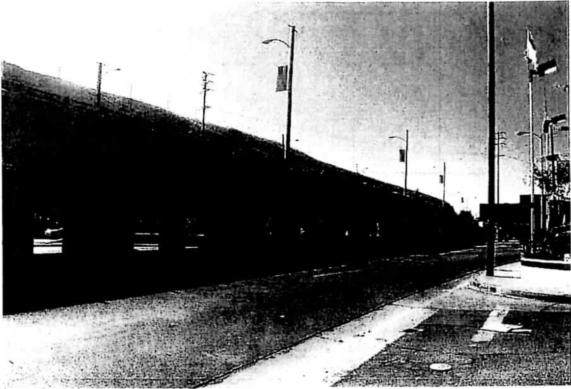
Soto Street Bridge over Mission Road and Huntington Drive Los Angeles, CA
