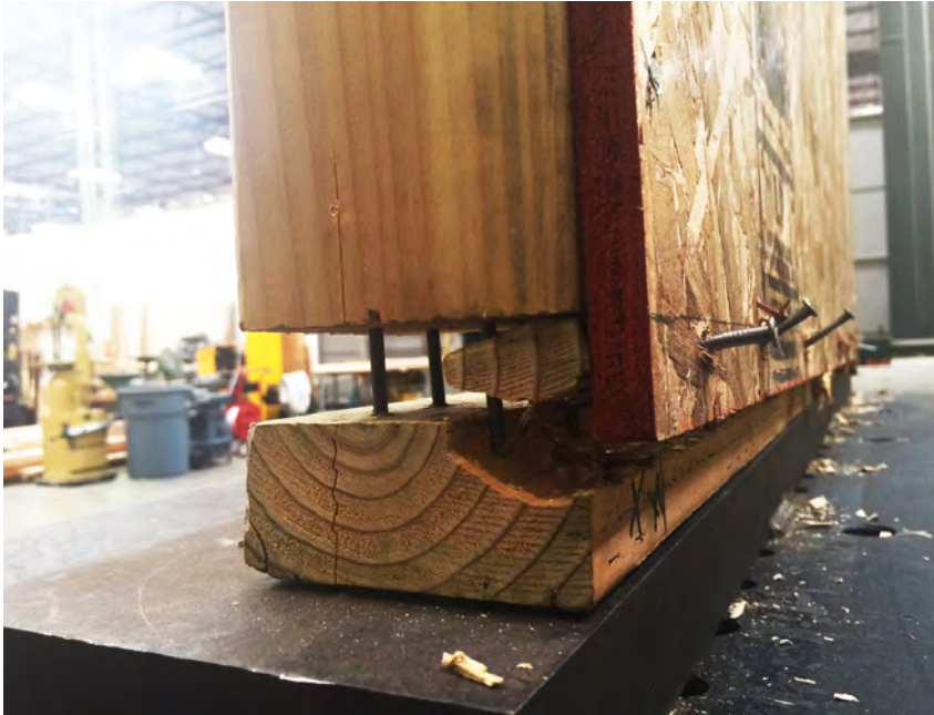
Sill plate split
