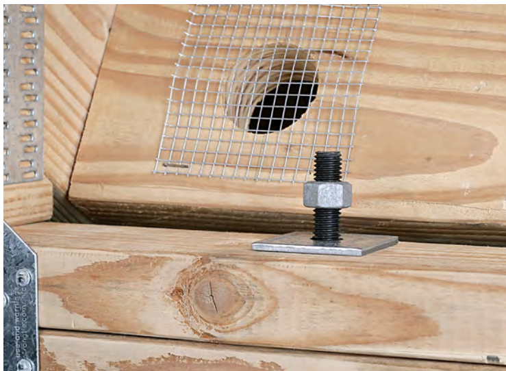
Gap between nut and bearing plate due to wood shrinkage.
