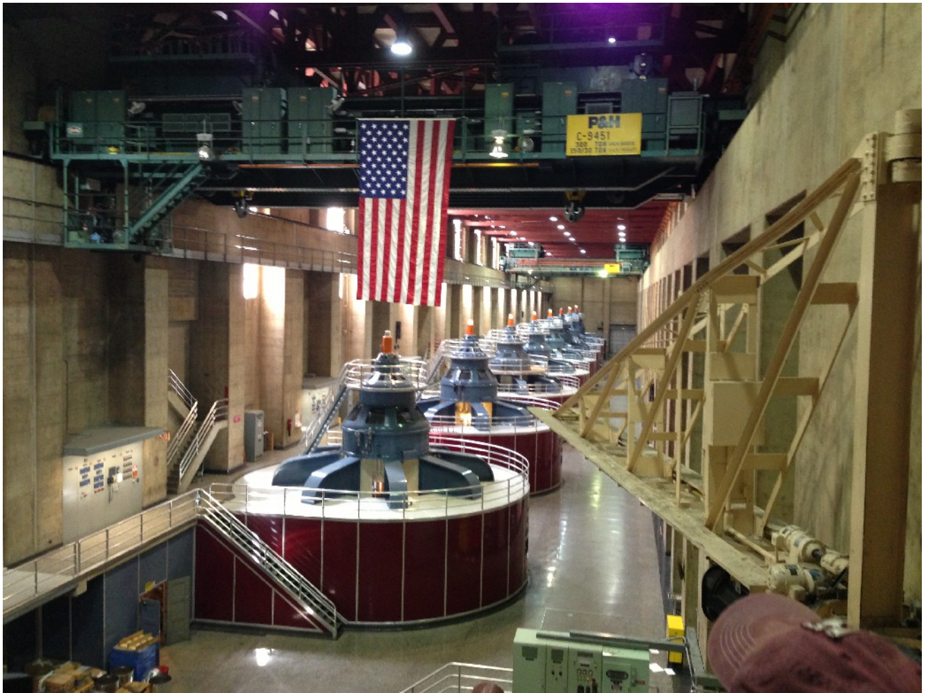
One set of generators.
