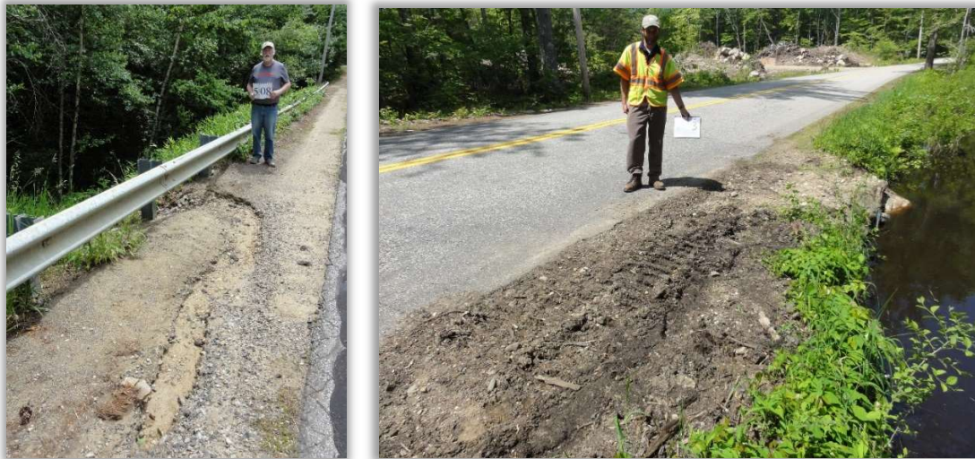
Top Left: Gully surface erosion, sheet/gully shoulder erosion, and unstable culverts contribute to this site's NPS pollution. Top Right: Rill shoulder erosion, unstable culvert, and bare soil contribute to this site's NPS pollution.
