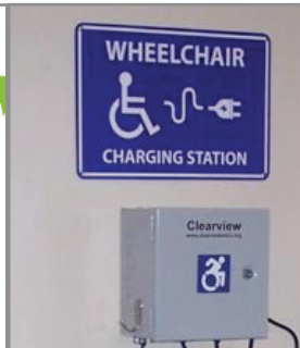
First Wheelchair Charging Station p.6
