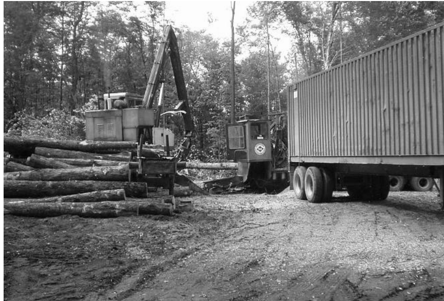
A whole tree chipper blows wood chips into a van so they can be trucked to an end user.
