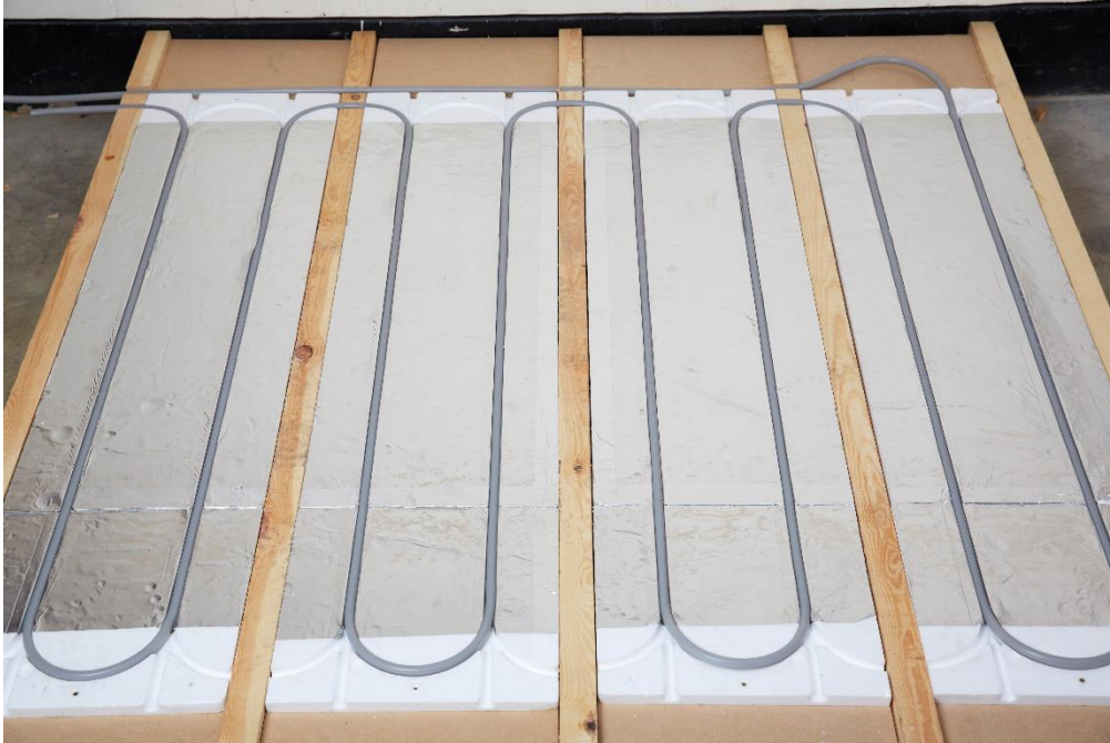
Low Profile Between the Joists
