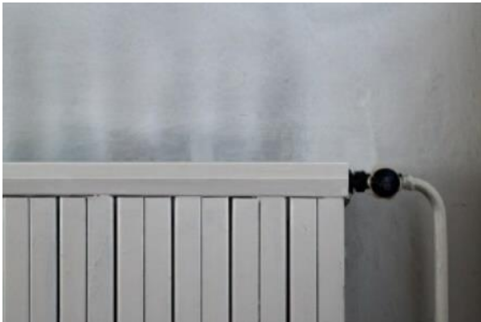
Radiator convection staining
