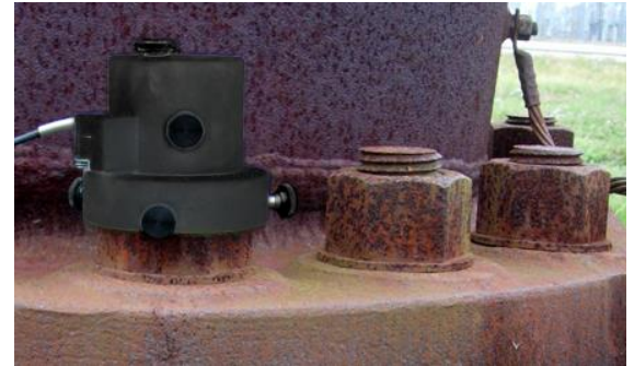
PAUT inspection with bolt scanner enables rapid data acquisition, permanent record and easy-to-interpret data analysis.
