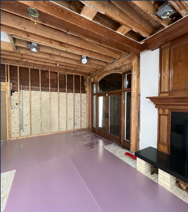
OPENED AND PROTECTED
