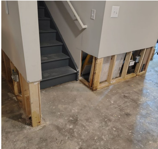
TWO-FOOT FLOOD CUTS
