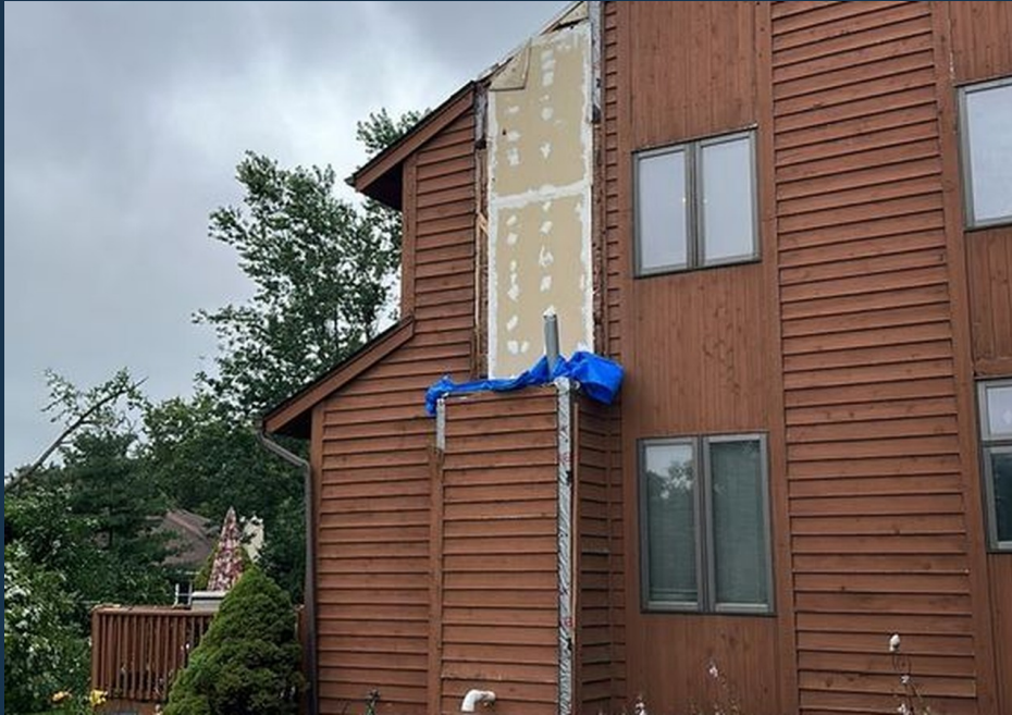
AFTER THE TORNADO
