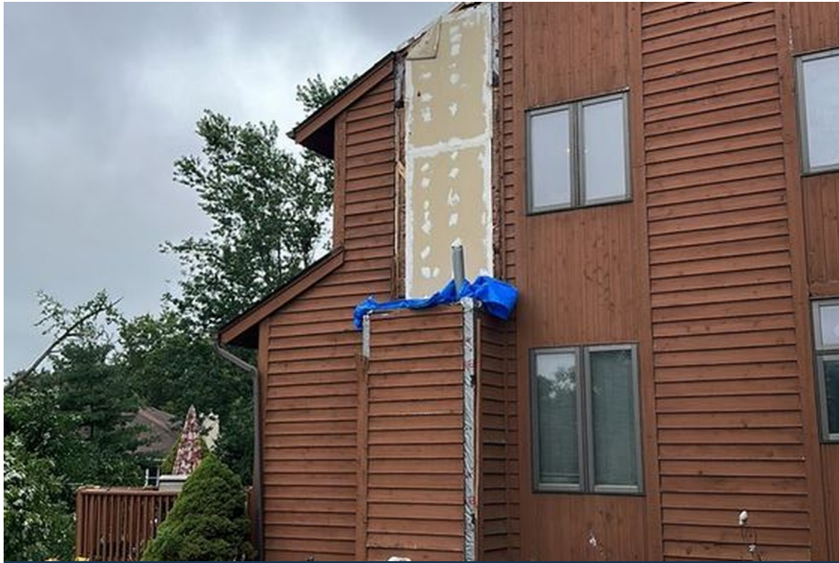
EXTERIOR DAMAGE DOCUMENTED
