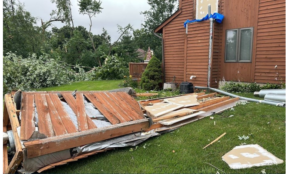
EXTERIOR ASSEMBLY DISPLACED
