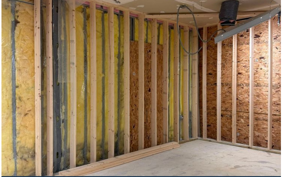
SUPPORT AND FRAMING CONDITIONS EXPOSED
