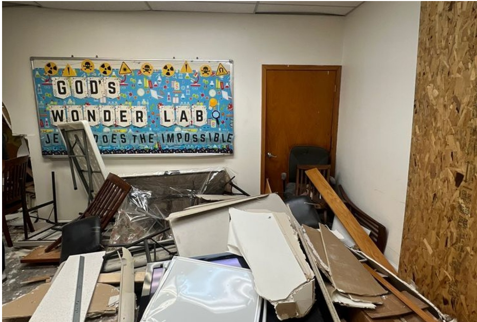
CONTENTS WITHIN THE DAMAGED AREA
