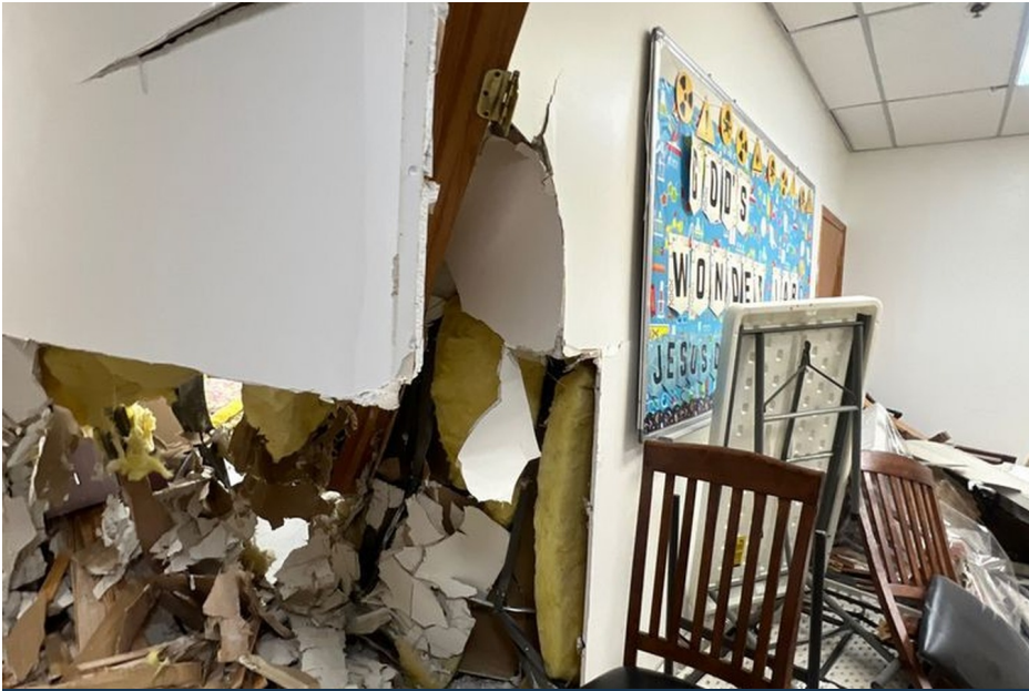
INTERIOR IMPACT AND DEBRIS
