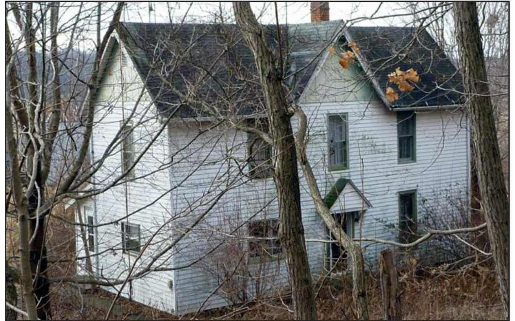
-Photo provided by the Indiana Division of Historic Preservation and Archaeology The home above is located on Hwy. 50 in Center Township. The house dates back to 1900. According to the survey results, the farmstead contains a brooder house, a drive-thru corner, and a summer kitchen.
