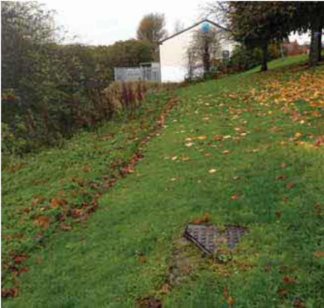
18) Drainage manhole in northern site area
