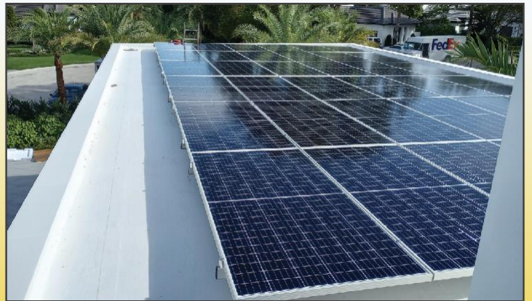
Close up of rooftop solar array on TPO style Kemper sealed roof
