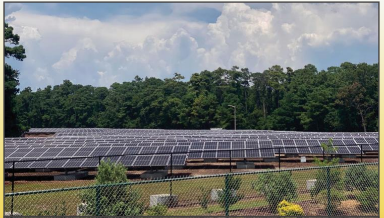
750kW Solar Farm, Cherry Hill, NJ
