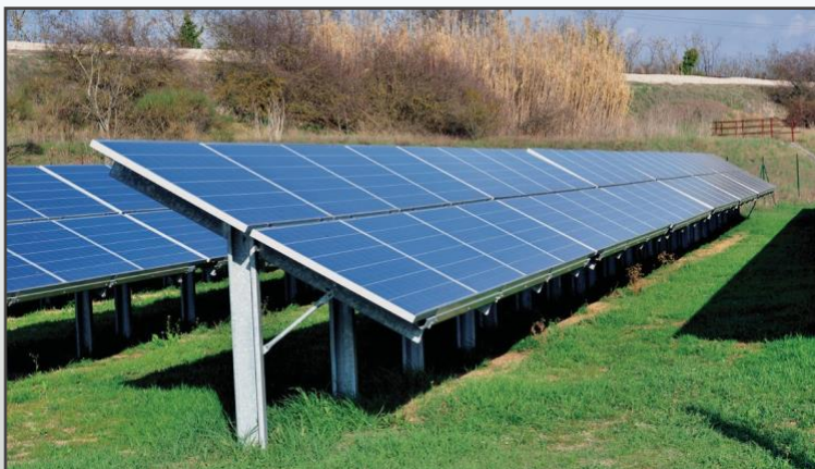
30kW ground mounted commercial system, Clermont, FL
