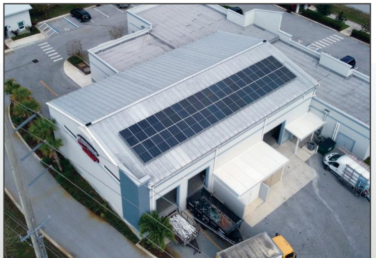
17kW commercial solar system, Stuart, FL
