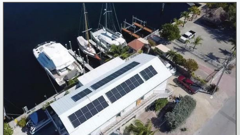
15kW Solar PV installation, Florida Keys
