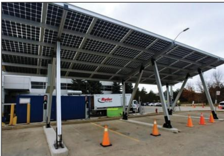
40kW Solar Carport, Orlando, FL
