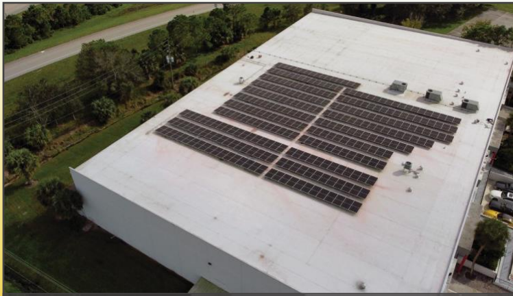
102kW Solar PV installation, Stuart, FL
