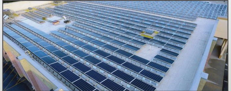
139kW Solar PV installation on retail facility, Tampa, FL
