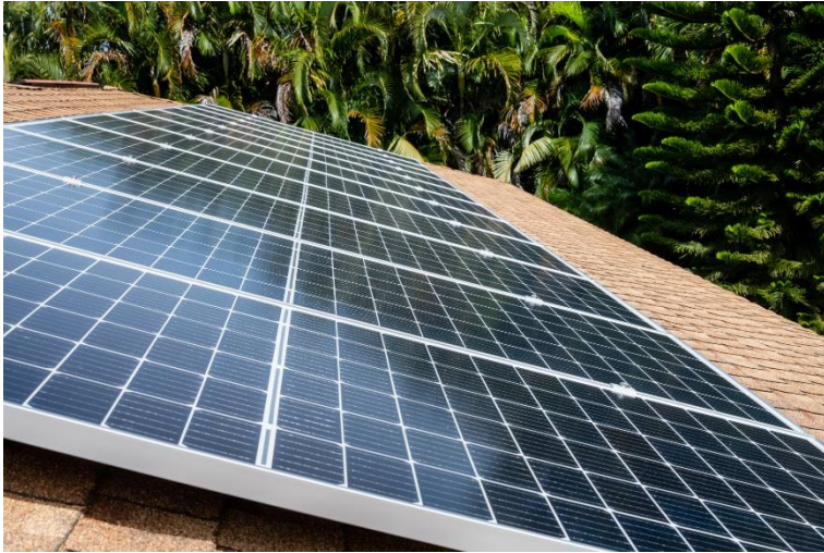
10.3kW Solar installation in Stuart, FL
