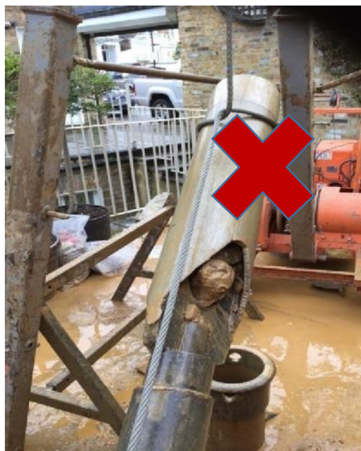
Incorrect use of wire rope to tip the Shell
