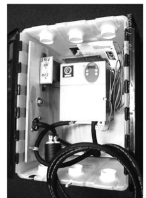
VFD mounted in box
