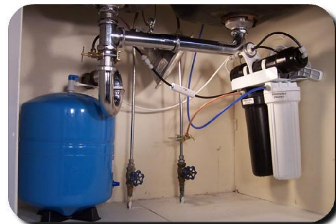
POU-RO Unit Installation
