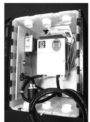
VFD mounted in box
