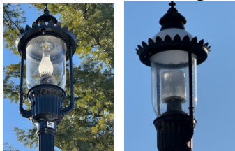
FIGURE 22: Ludlow Avenue 's Retrofit LED Streetlights
