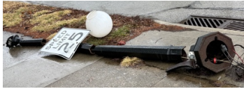
The fractured cast iron post
