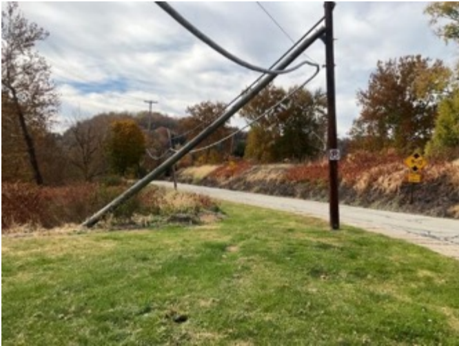
(E) CT8. Overhead lead sheathed cable running across a greenway and sidewalk. February 2023. Coal Center, Pennsylvania.
