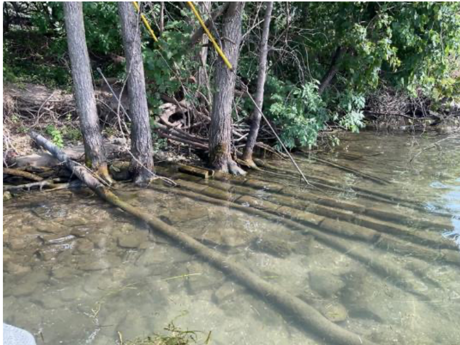
(C) Seven lead sheathed cables in the Detroit River. DR 1. July 2022, Trenton, MI.
