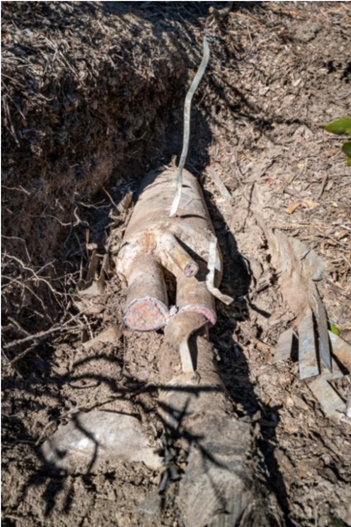
(A) Severed lead sheathed cables, and lead splice box on land. This photo was during a site visit with AT&T in January 2021.
