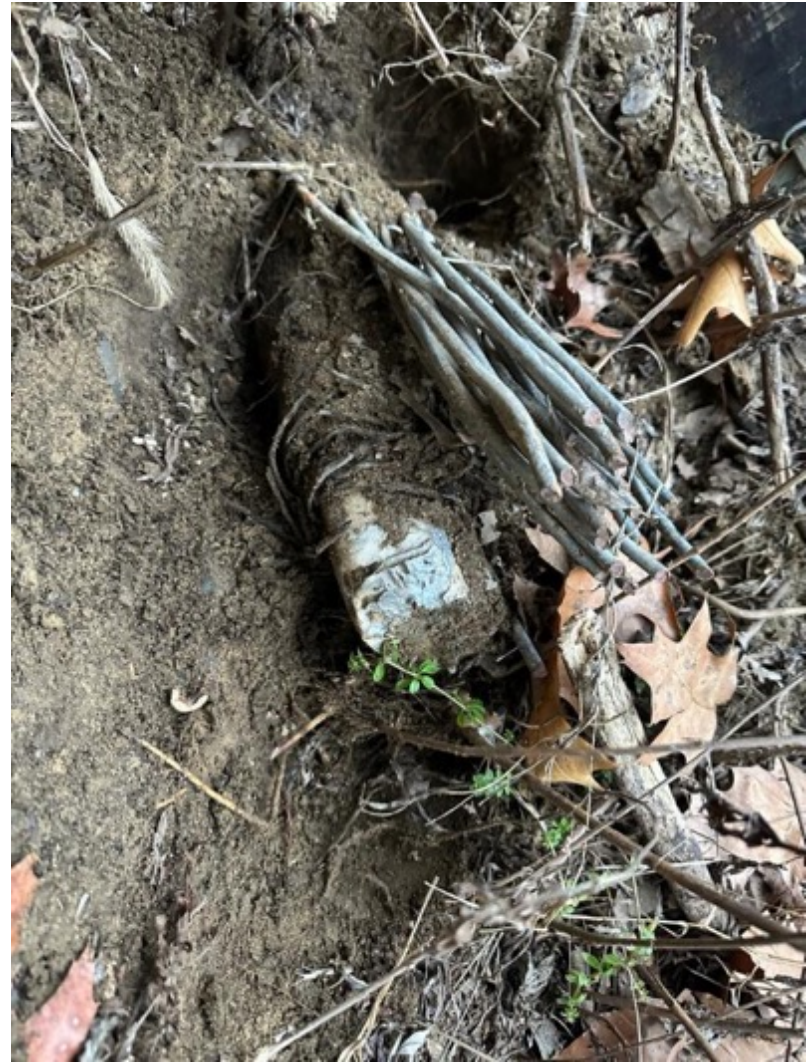
(E) Severed cable and steel wire at the base of an old telephone pole, across from those shown in (D). Point if Interest: Hudson 3.4. January 2023. Highland, New York.
