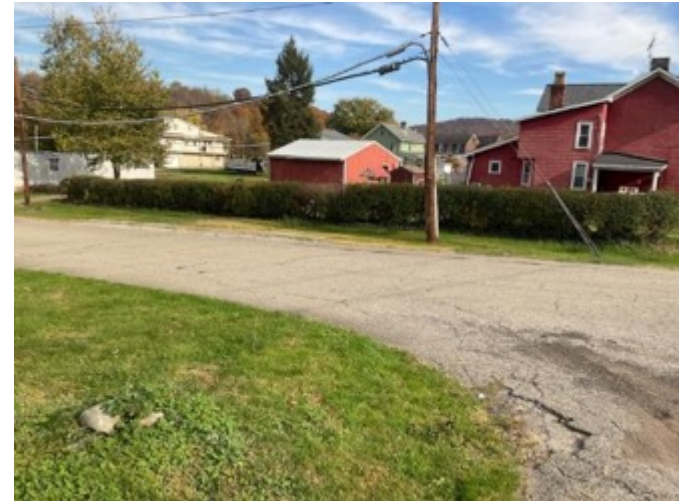
(G) CT12. Overhead lead sheathed cable running across the road next to homes. October 2022. Coal Center, Pennsylvania.
