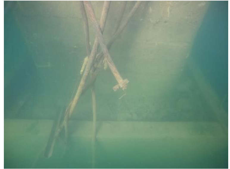
(B) Photo. Lead sheathed cables just below the surface. Site LP 4.1. August 2022, Lake Pend Oreille, ID.
