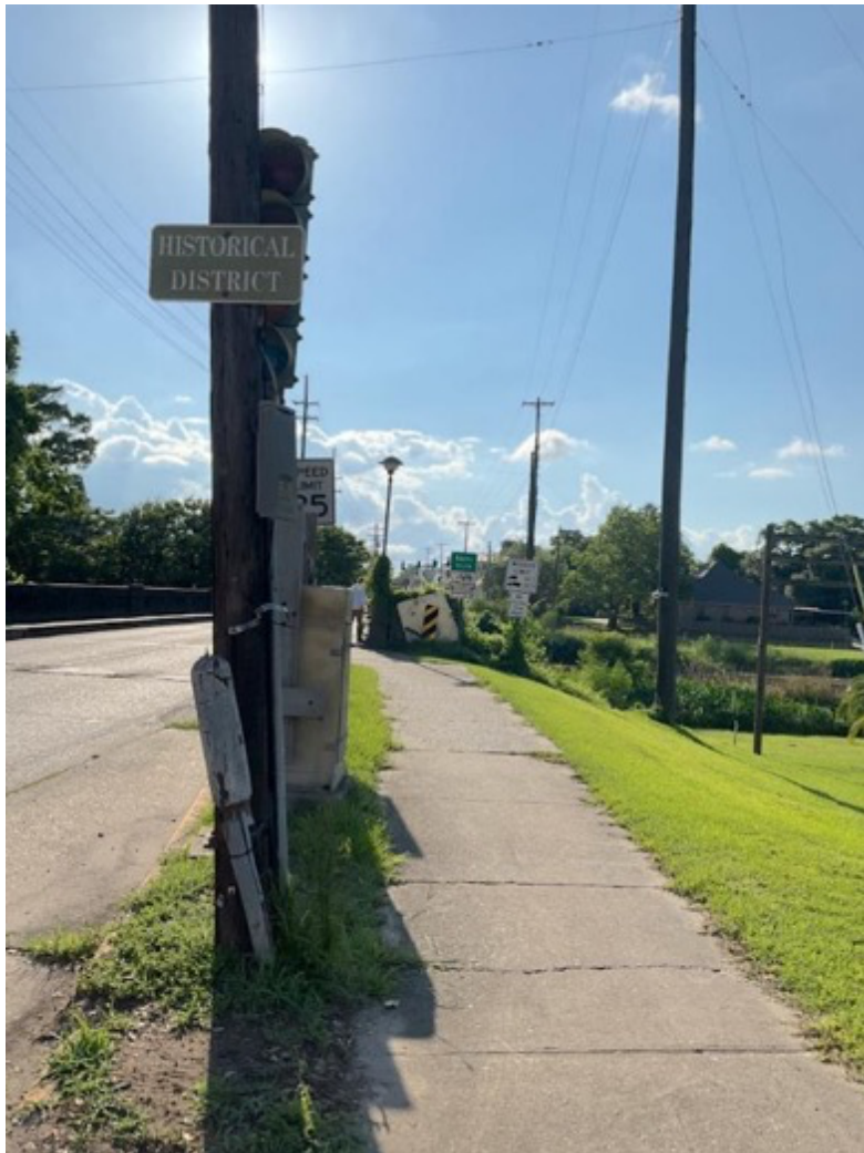
(G) Bare lead sheathed cables going into a lead splice box near the sidewalk leading into the Historical District. BT 24.1. June 2022, St Martinville, Louisiana.
