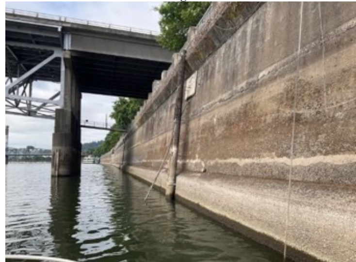
(D) Smaller lead sheathed cable below Western Union Telecom Co. Sign. WR 3. August 2022, Portland, Oregon.
