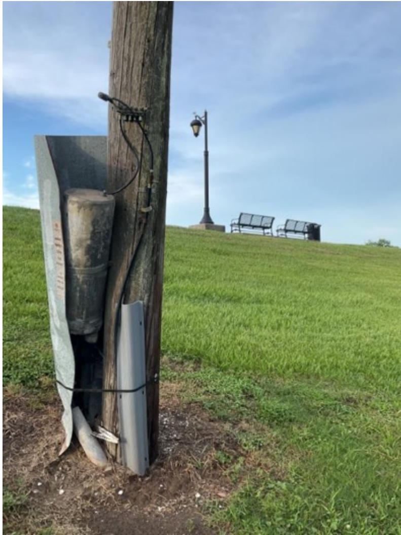
(M) Donaldsonville, LA. Location MISS 12.1. Exposed leaded splice box that appears to still be connected to an air test line. See photo (L) for the abandoned cable just the other side of the splice box. June 2022,
