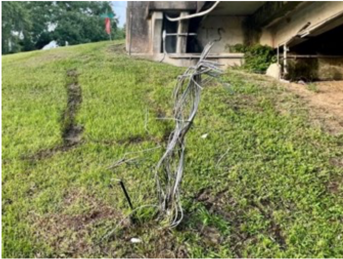
(C) Remnants of bare lead sheathed cable and steel wire below the Bridge Street Bridge. BT 1.1. June 2022, New Iberia, Louisiana.
