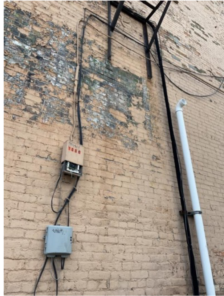
(B) End of the lead sheathed test line shown in (A). LH 2.3. July 2022, Bay City, MI.
