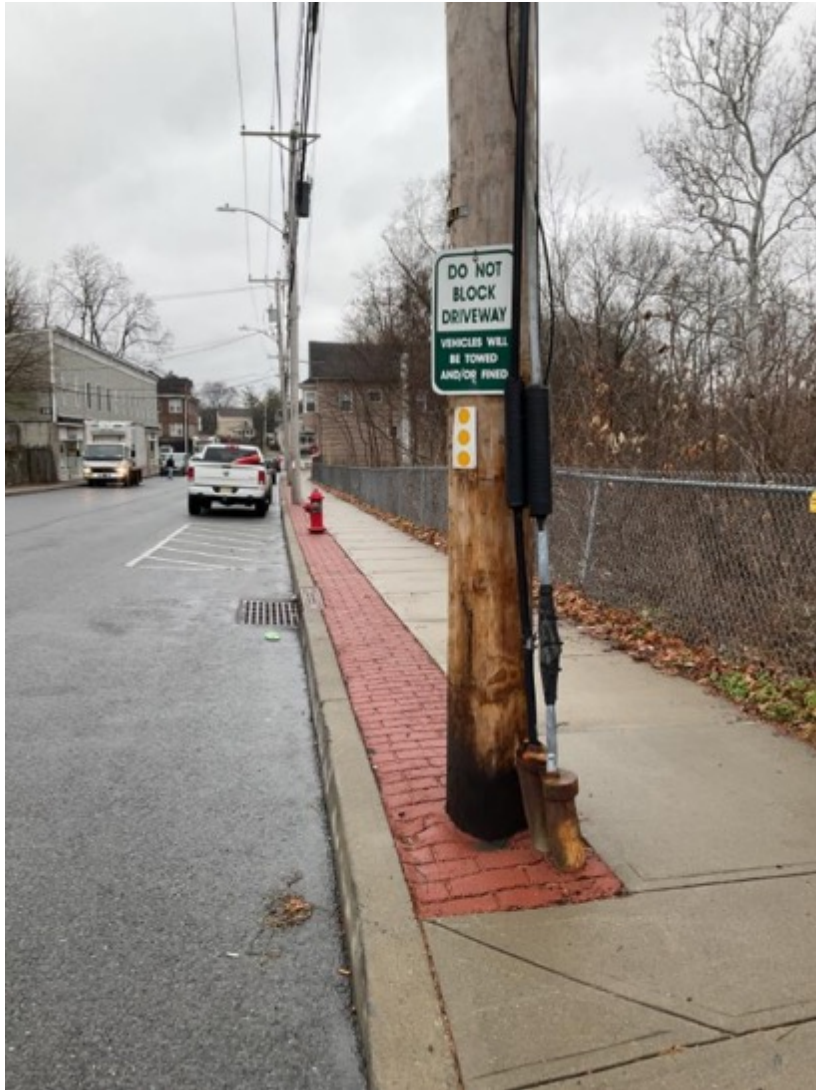
(K) Damaged lead sheathed cable at the base of a telephone in Wappingers Falls. Point of Interest: Wappingers Falls 3. January 2023, Wappingers Falls, New York.
