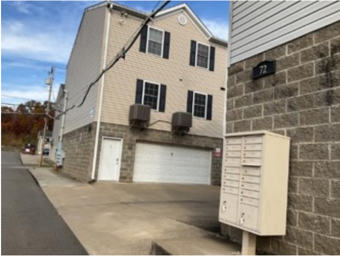
(D) CT6. Overhead lead sheathed cable running across the entrance into apartments and over access to mailboxes. February 2023. Coal Center, Pennsylvania.
