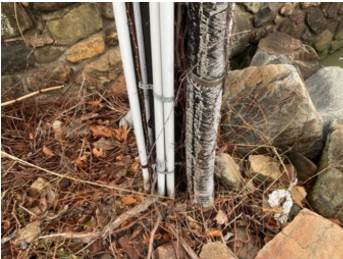
(I) Close up of abandoned 5" lead sheathed cable along the Hudson River. January 2023, Palisades, New York.
