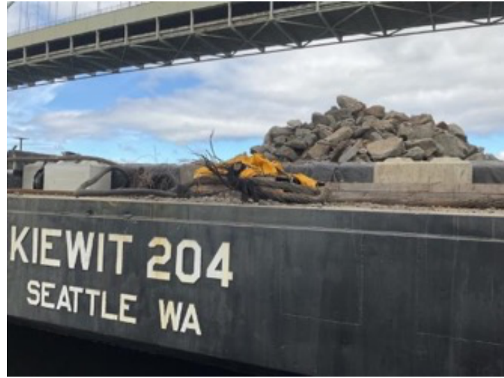
(G) Active construction site. Lead sheathed cable. Kiewit 204. WR 8. August 2022, Portland, Oregon.
