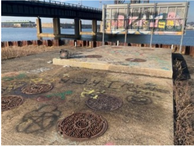
(A) Large vault with eight Bell Systems manholes on the Hackensack River. Looking towards South Kearny. January 2023, West Side, New Jersey.
