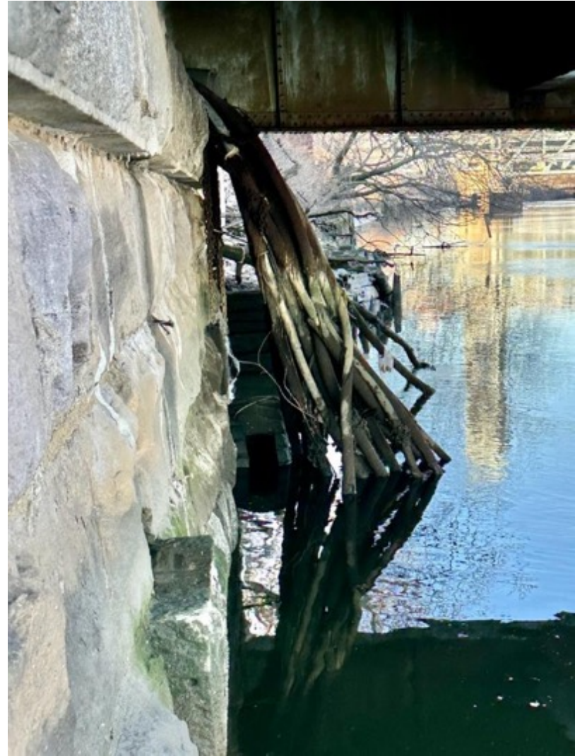
(I) Cable location with twenty lead sheathed cables underneath the Bridge Street Bridge (Harrison Ave.). Passaic 2.1 January 2023. Harrison/University Heights, New Jersey.
