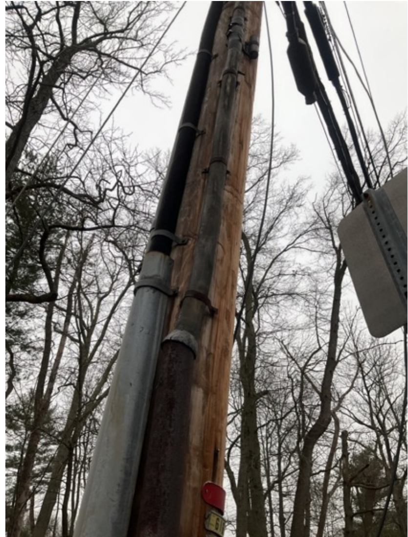
(J) Bare lead sheathed cable running up telephone pole in the Palisades. January 2023, Palisades, New York.
