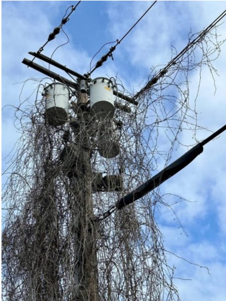
(F) “Squirrel Guard” tied around an exposed area of lead sheathed cable. Point of Interest: Newburgh 1. January 2023, Newbury, New York.
