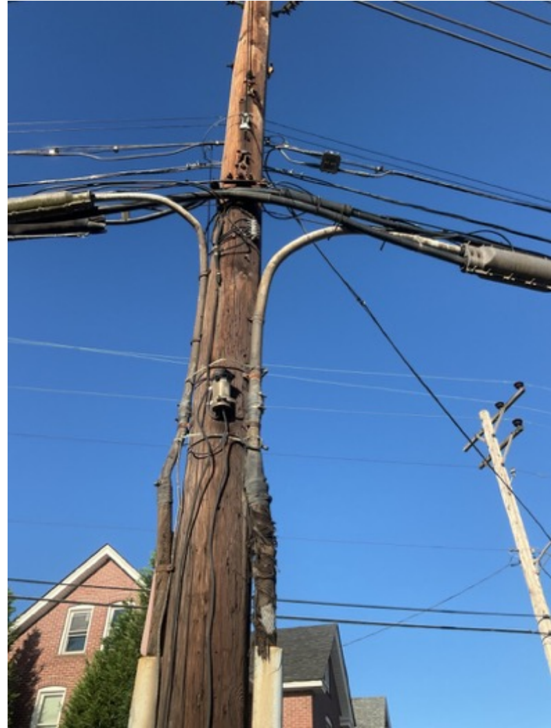
(C) Close up of lead sheathed cable and splice boxes referenced in (A). October 2022. Natrona, Pennsylvania.
