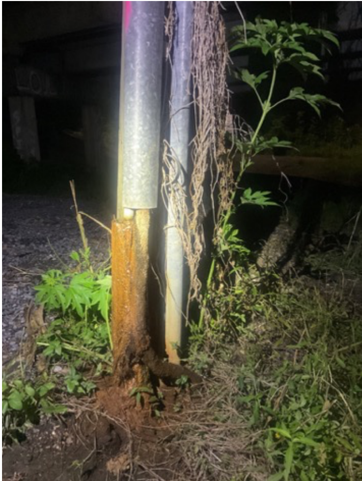
(B) Old telephone pole with cable guard and old conduit where a cable would have been. There is currently corrugated plastic hose behind the guard and in the steel pipe, but no visible cable. BL 2.2. Labadieville, Louisiana. June 2022.
