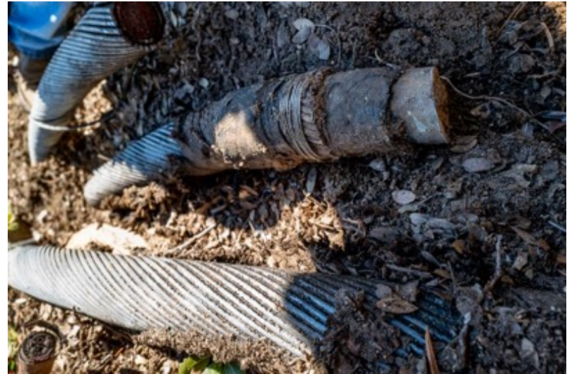
(B) Another splice location from land during the same site visit with AT&T in January 2021.
