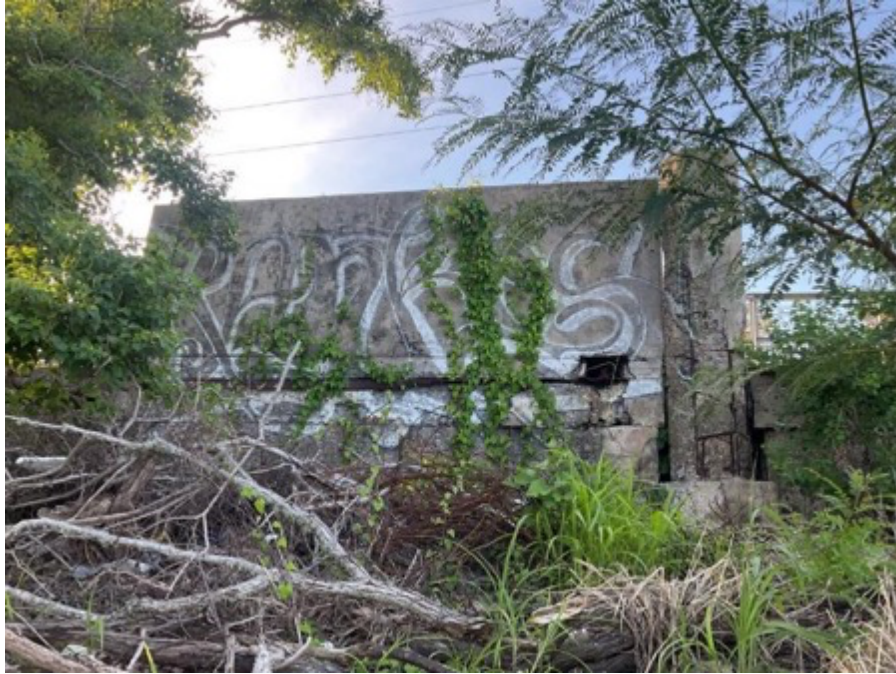
(K) New Orleans, LA. MISS 3.1. The small rectangle on the left is the passthrough for utility cables. June 2022.
