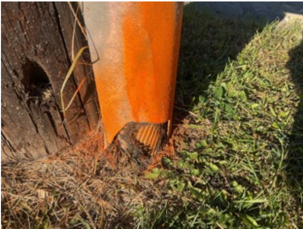
(B) Base of telephone pole in (A) and (C) showing marked cable going into the ground. October 2022. Natrona, Pennsylvania.
