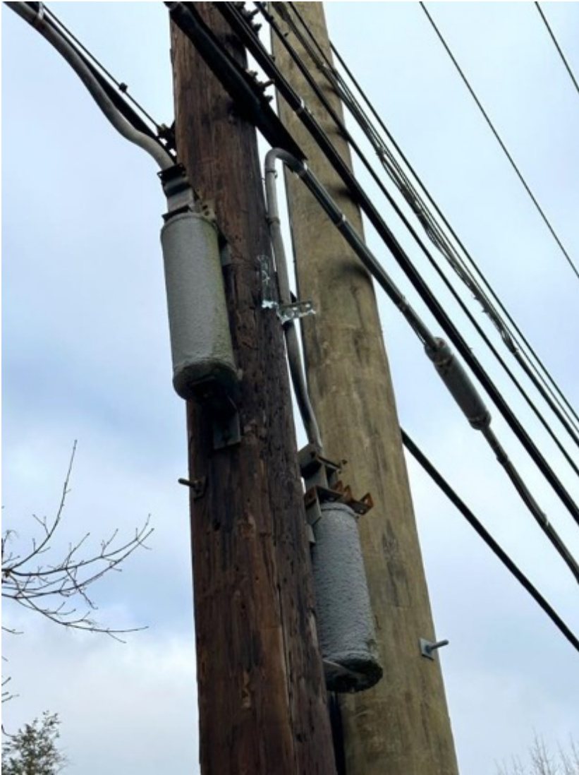
(A) Close up of telephone poles with overhead lead sheathed cable and leaded splice boxes. January 2023. Highland Falls, New York.
