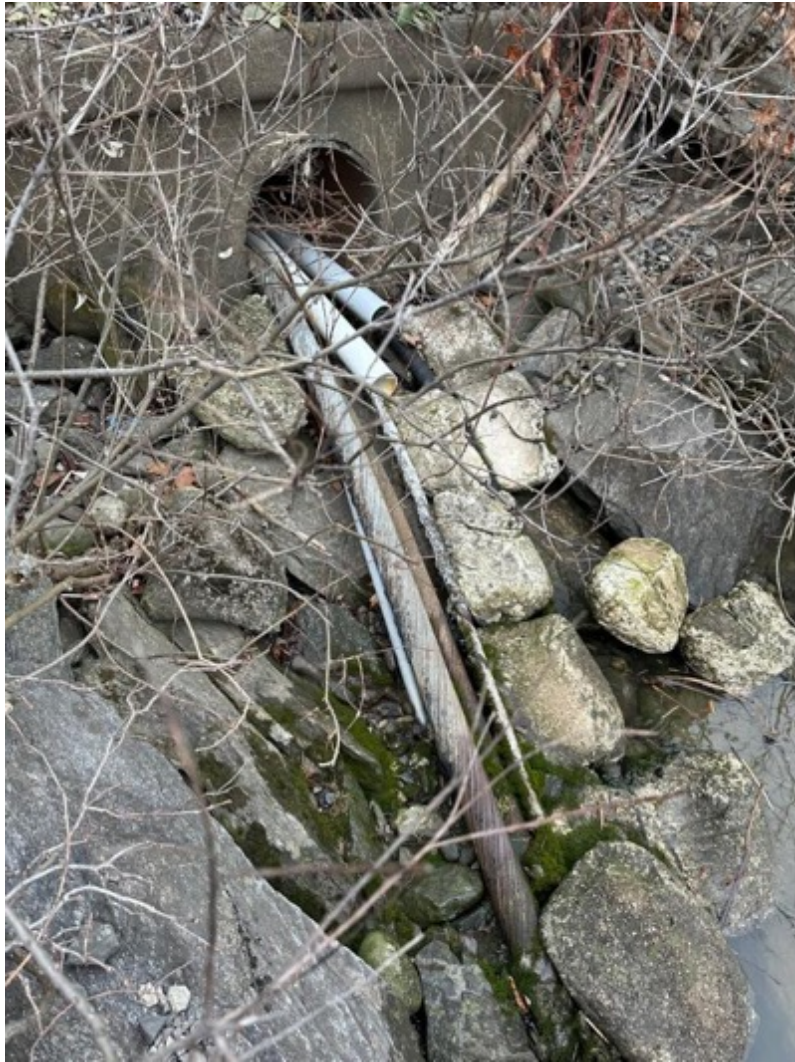
(D) Cables run under the road and into the Hudson River near the Mid-Hudson Bridge at Point of Interest: Hudson 3.1. January 2023. Highland, New York.
