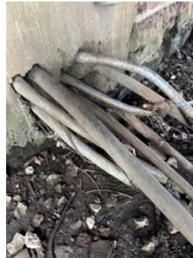
(L) Part of an eleven-cable location found near Wall Street Bridge, between Garfield and Wallington. Passaic 8. January 2023. New Jersey.
