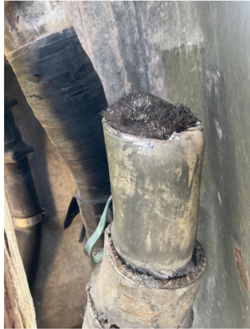
(N) Donaldsonville, LA. Location MISS 12.1. Close up of lead sheathed cable next to lead splice box seen in (K). June 2022.
