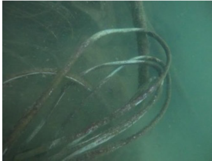
(G) Close up of bare lead from abandoned cables. Site LP 4.1. August 2022, Lake Pend Oreille, ID.
