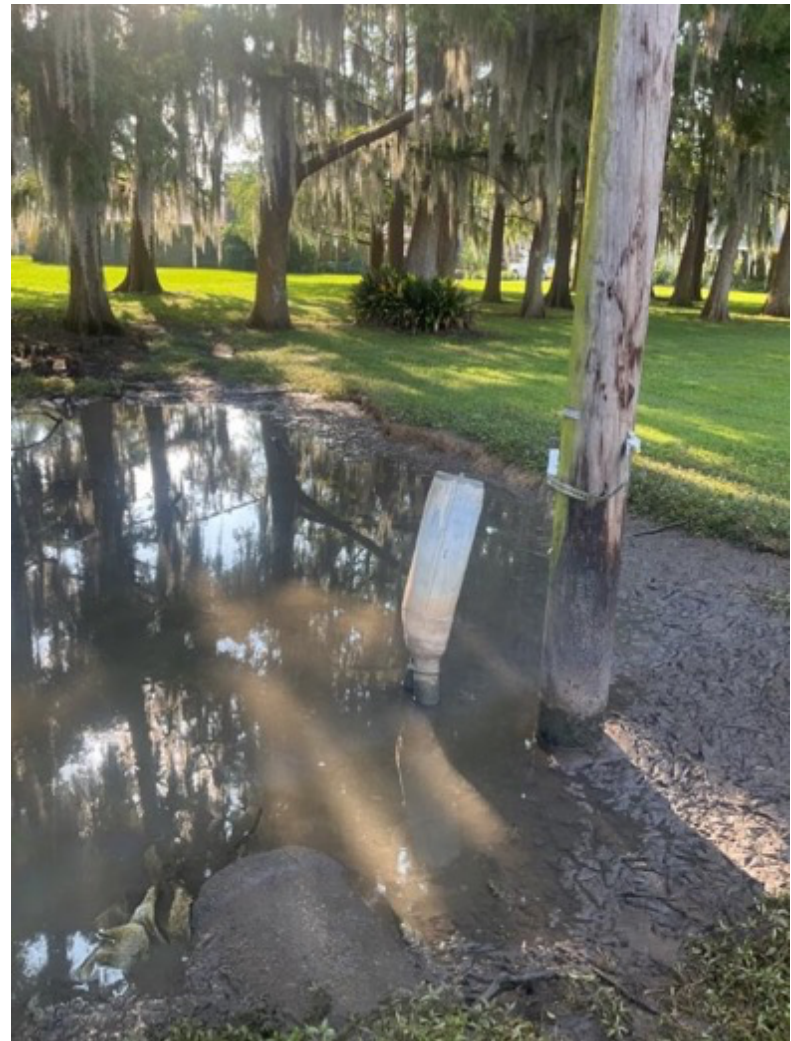
(H) Exposed lead splice box with attached cables and drainage into the Bayou Teche. BT 26.2. June 2022, Franklin, Louisiana.
