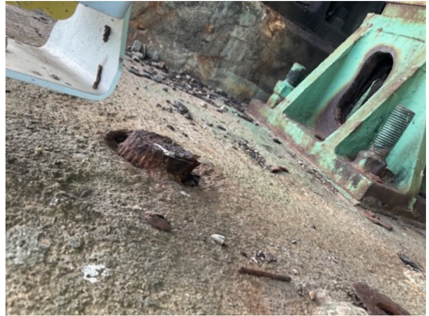
(F) Cut lead sheathed cable, referenced in (E). DR 2. Grosse Ile Township, MI.
