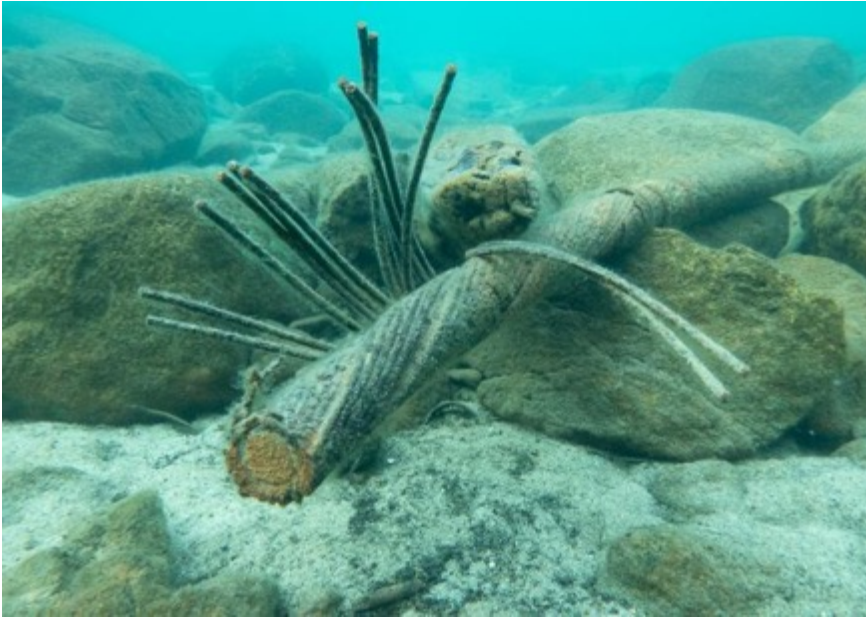
(G) Severed end of 1920's cable in Emerald Bay. May 2021, Emerald Bay - Lake Tahoe, California.
