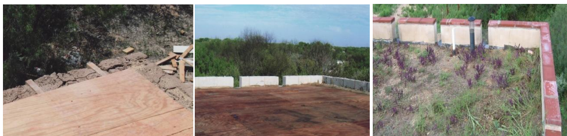
Figure 4. Construction the Mexican green roof: Left: 2 x 12, emplaced on concrete bond beam with \frac{3}{4} inch plywood decking. Center: Cinder blocks (CMUs) are used for parapets; gaps for canals. Right: Membrane, canals and soil emplaced.
