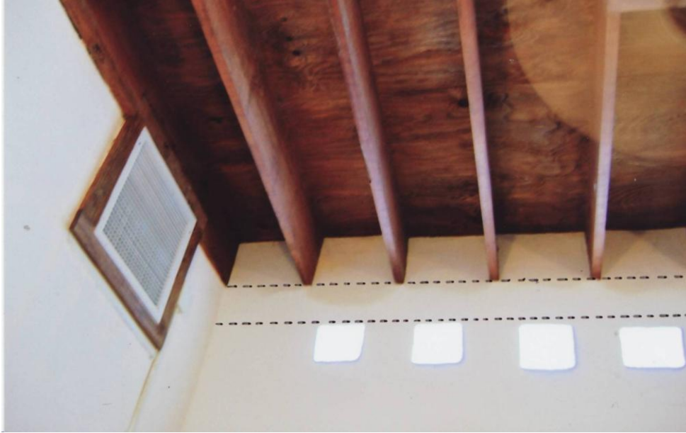
Figure 5. Room interior with the Mexican brown roof (no vegetation). Ceiling is also the decking; 2x12 inch timber on bond beam noted by dashed line.
