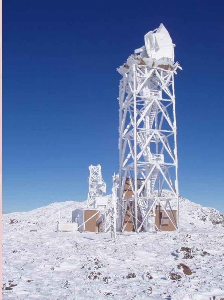
Figure 4-4 NWS Reno Radar Damage from Wind (December 2008)
