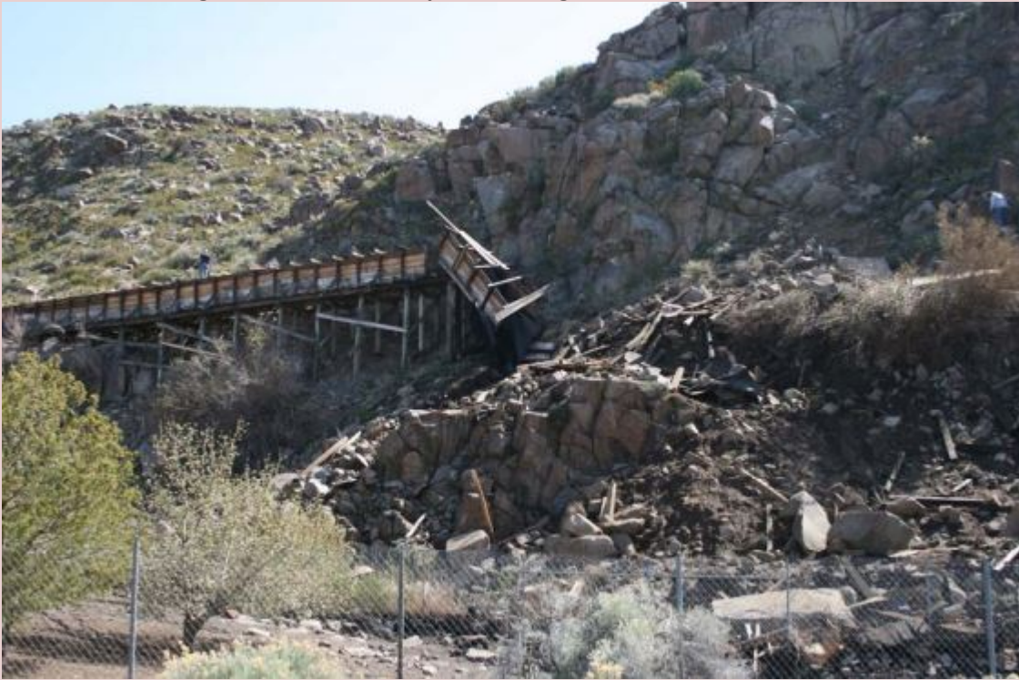
Rock fall damage to water flume
