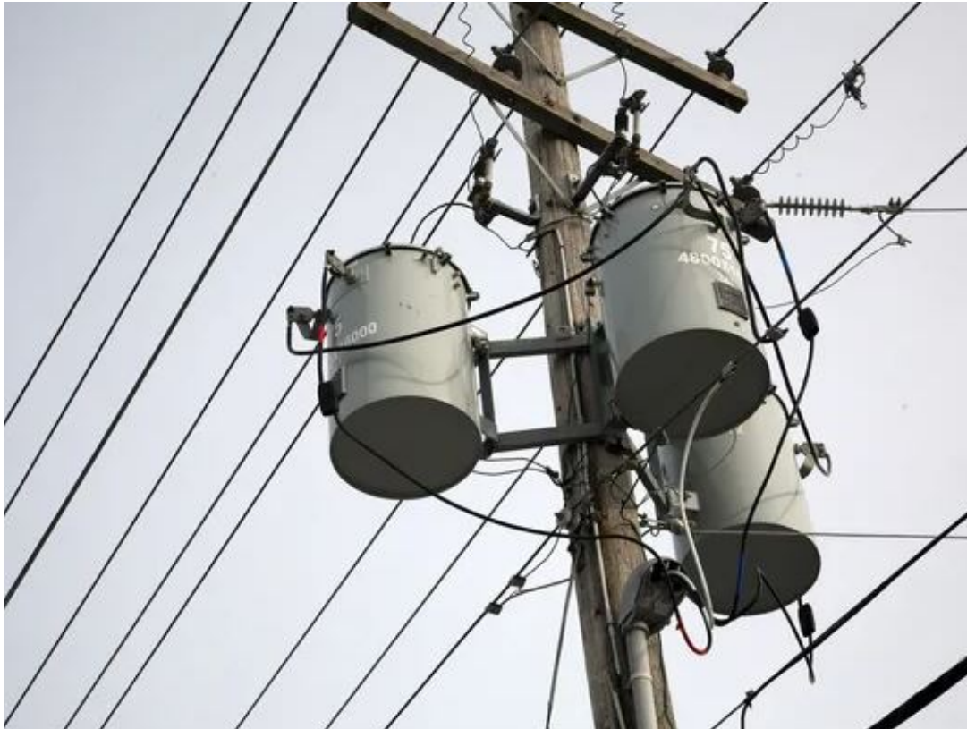
Utility pole with power lines and transformers.
