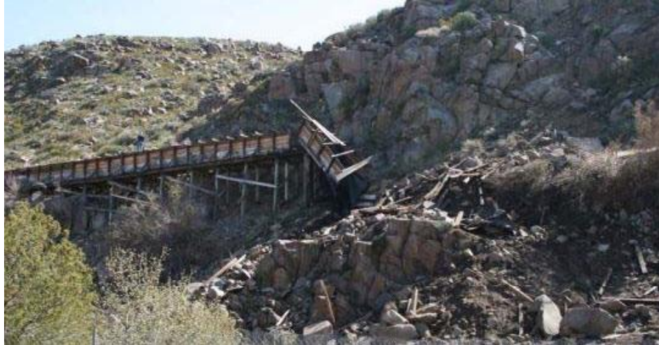
Figure 47: Water Flume Damaged by the Mogul–Somerset Earthquake, 2008 97
