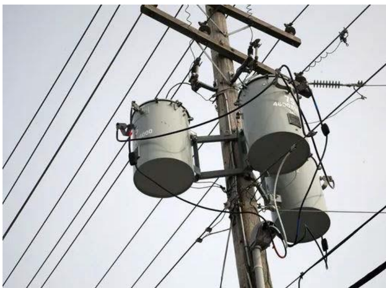
Figure 77: Utility Pole with Power Lines and Transformers 120
