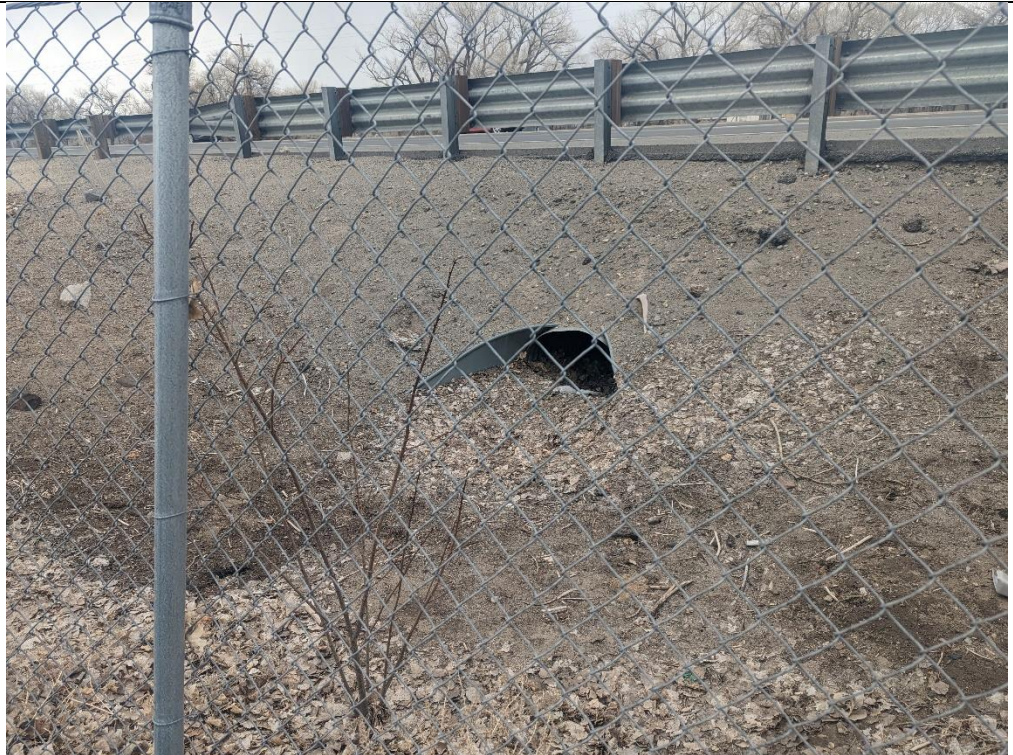
Photo 6. Image of the Our Park drainage imaged in the previous FYR that had erosion issues potentially exposing the sub cap materials.
