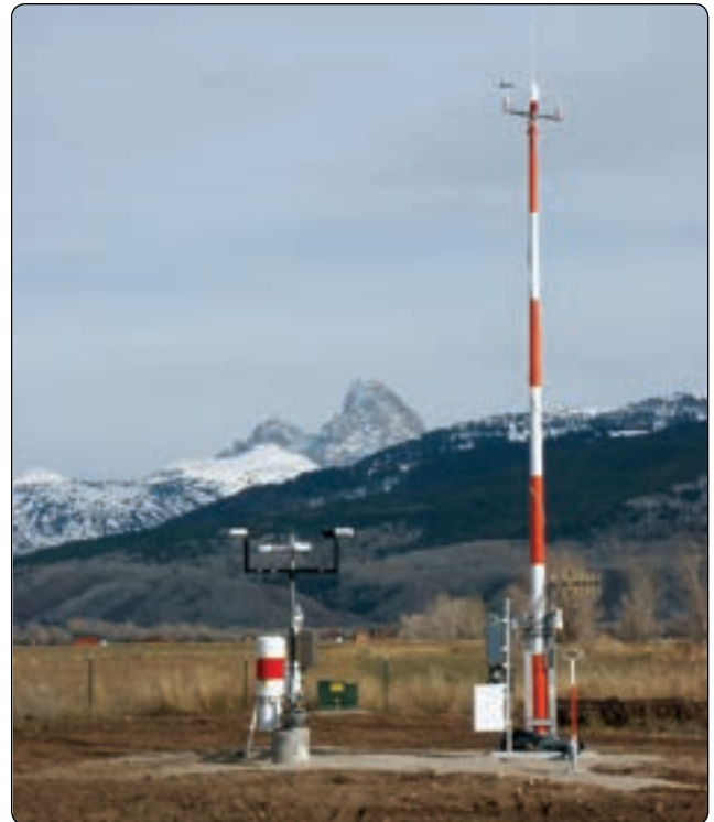
Figure 1-11. AWSS installation at Driggs-Reed, Idaho.
