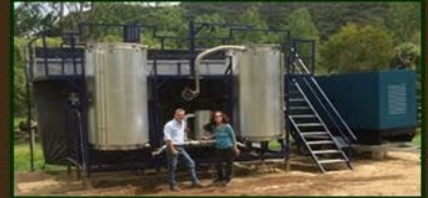
2021 - extraction plant, commissioned/ready
