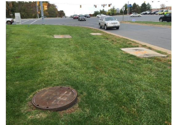
Hand holes are concentrated near the intersection of Waxpool Road and Pacific Boulevard
