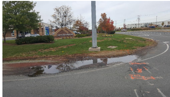
The northwest corner of the intersection lacks a curb ramp and curb and gutter infrastructure
