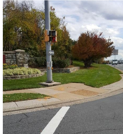
Some existing ramps require upgrades
