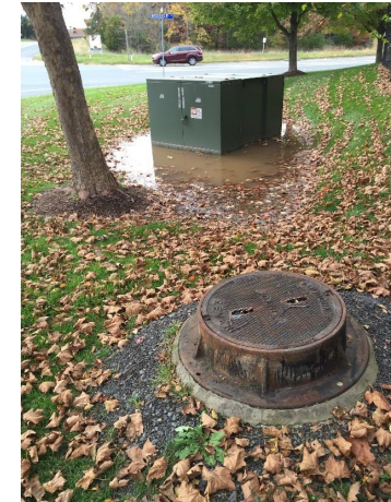
Ponding around a transformer near the proposed corridor for sidewalk on the north side of Prentice Drive
