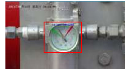
Broken of facilities
