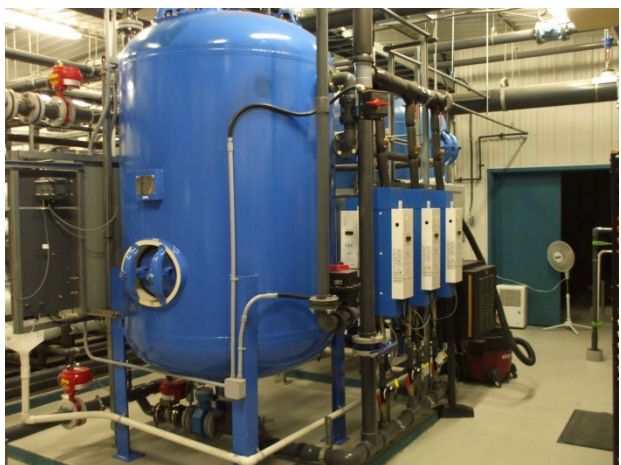
The New Sand Filter with UV
