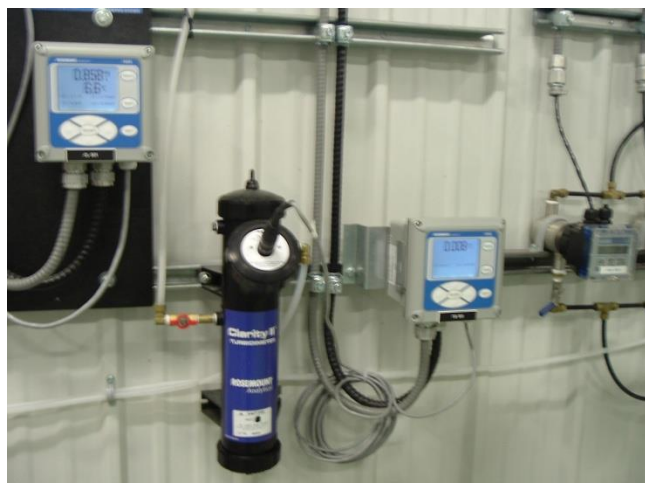
Online Monitoring Equipment
