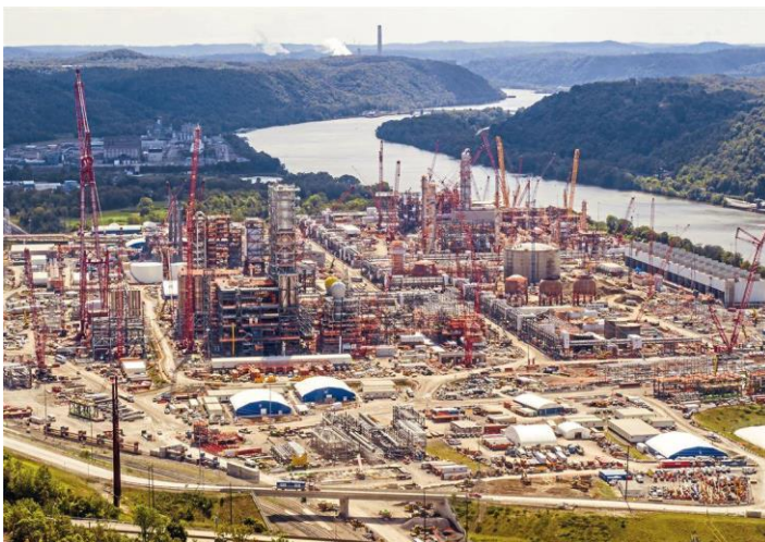
Image 2: Shale Gas Buildout in the Appalachian Basin, 12/8/19 Courtesy of Concerned Ohio River Residents.
