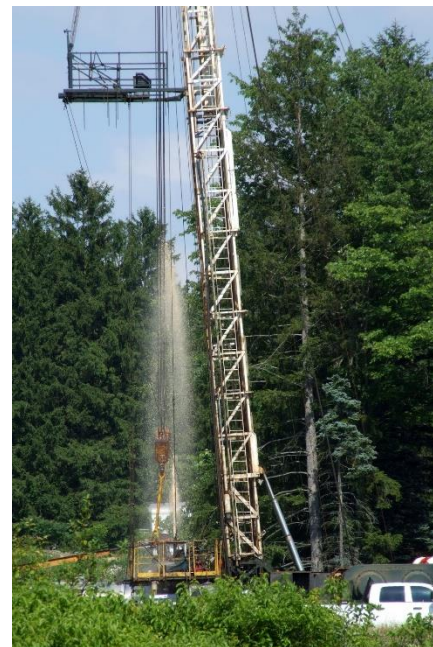
Image 1: Injection Well in Southeast Ohio
