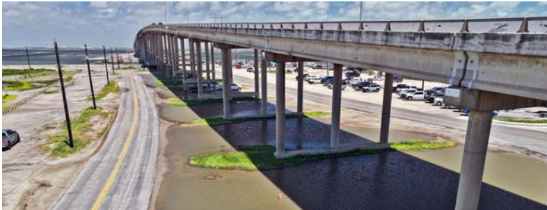
It is all water under the bridge after every rain under the causeway
