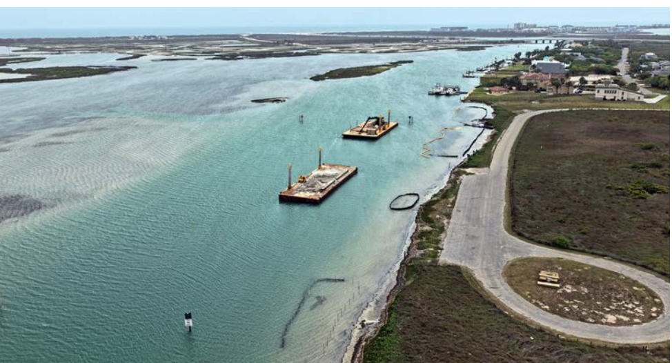
Location of the new fishing pier with the 361 bridge in the background
