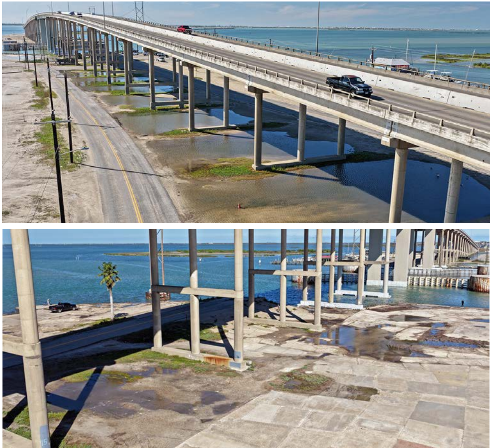
The areas under the JFK Causeway "Muddle and Puddle" filled up with water after our Easter rain last week. Plans to fill the low areas are in the works.
