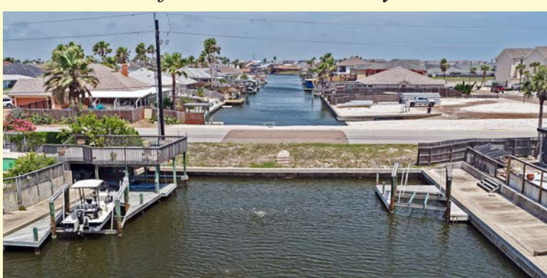
History cont. on A5 The Encantada culverts are filled with sand. Bubblers were installed on one side to aerate stagnant water
