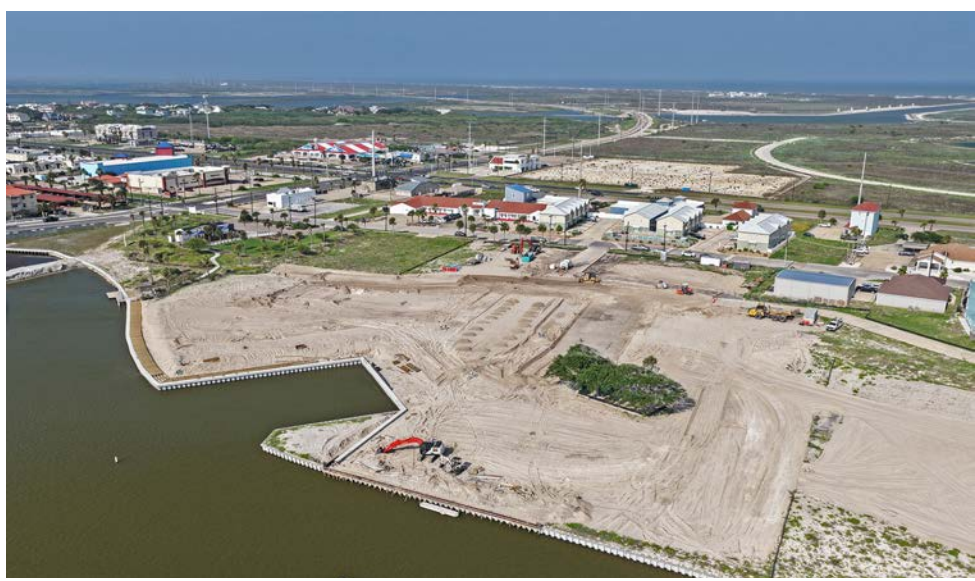
The Early Activation Area at Whitecap NPI is under construction. The area will serve as a social area for events like the Farmer's Market, and will be the first phase of commercial and retail development in the project. They will have dock space available for boat parking.
