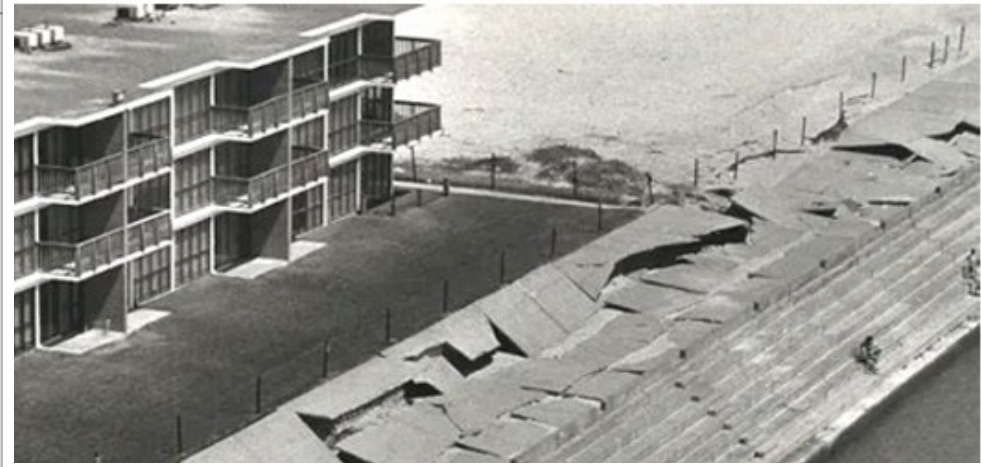
Michael J. Ellis Seawall after Hurricane Allen in 1980
