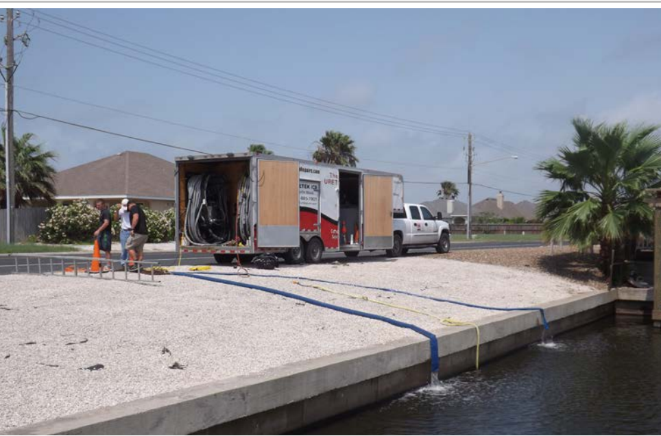
Ten years ago in the Island Moon. Work continues to repair and open the water exchange tubes under Encantada.
