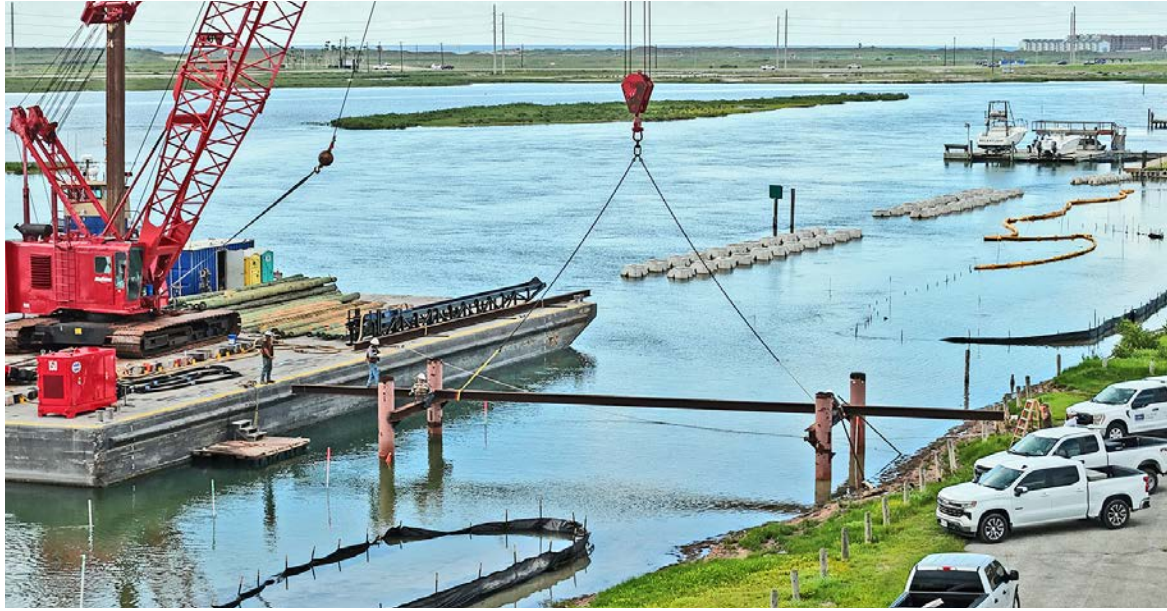
Work continues at Packery Channel Park as crews continue installing the living shoreline. The park is closed while under construction, and when it reopens will feature a fishing pier.
