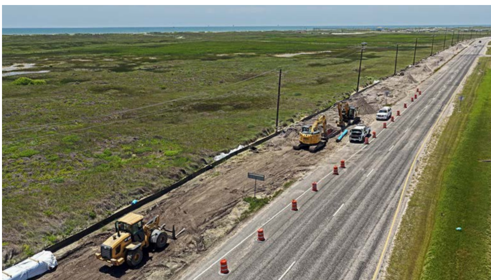
Work continues on the water line going in south of Whitecap on Park Road 22
