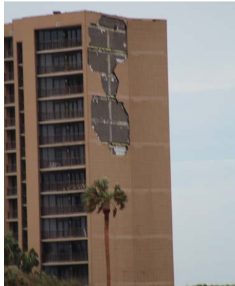
Damage to the exterior of the Sandpiper Condos
