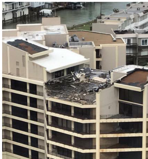
Damage to Clines landing
