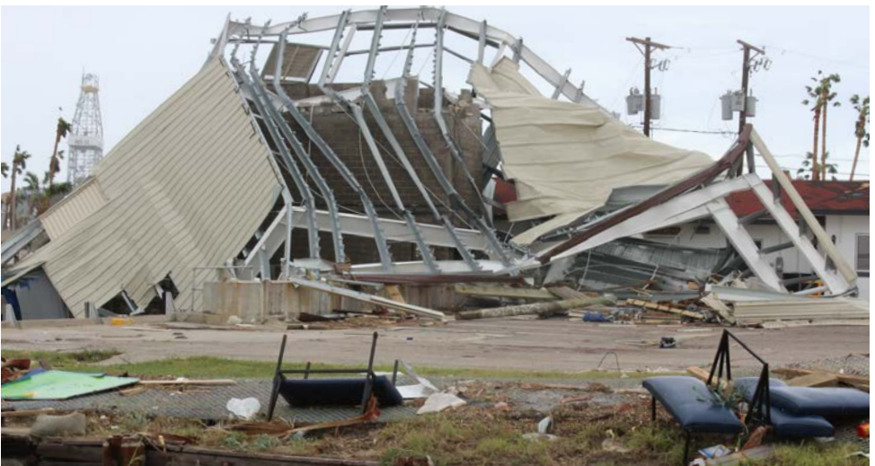
Metal buildings did not fare well
