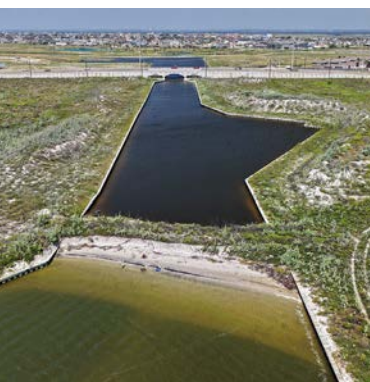
The sand dam blocking water flow under the Don Patricio Bridge
