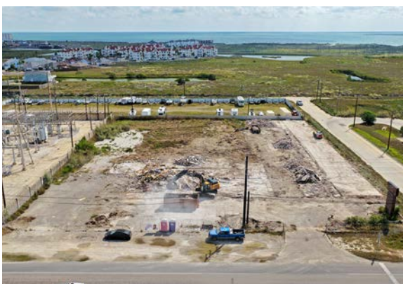
The Island Italian and hotel property this week as part of the expansion of the AEP Substation
