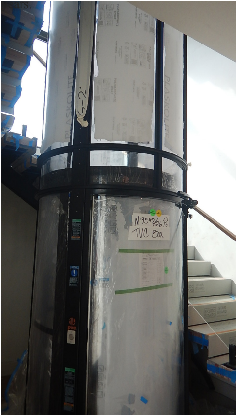
Whitecap NPI Model home interior elevator
