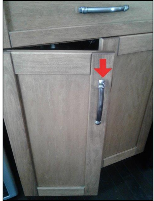
35. Pieces missing or loose
