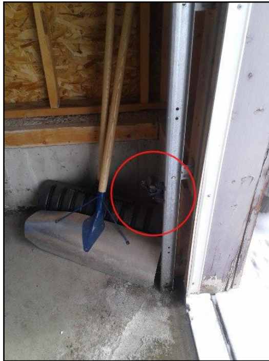
20. Sensors poorly located
