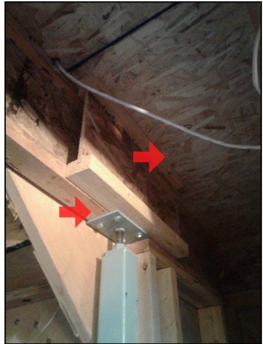
22. Weak connection to joists
