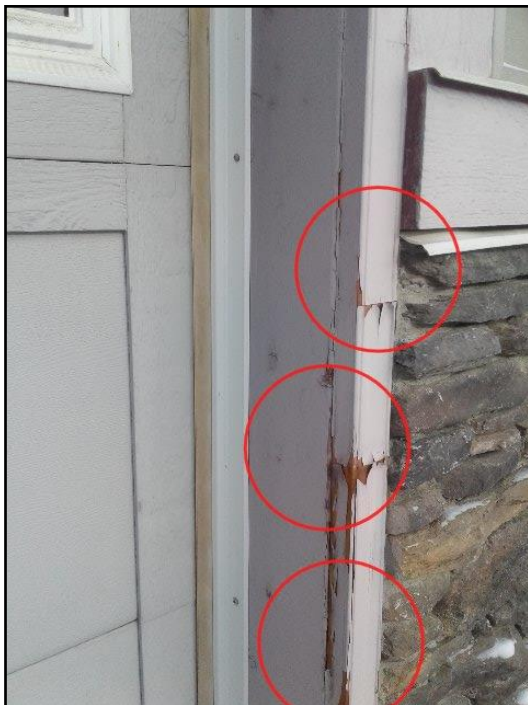
17. Paint or stain needed
