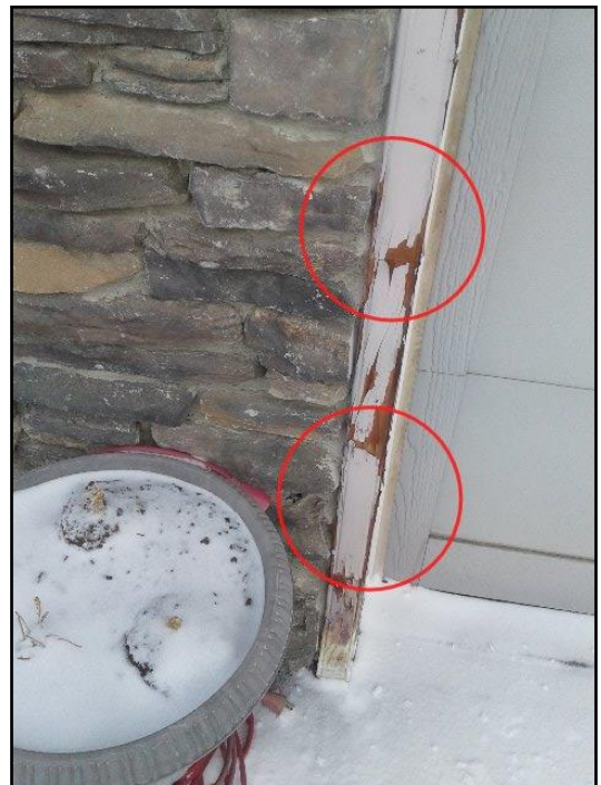
18. Paint or stain needed
