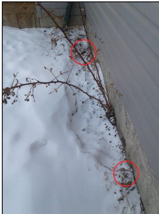
19. Improper slope or drainage
