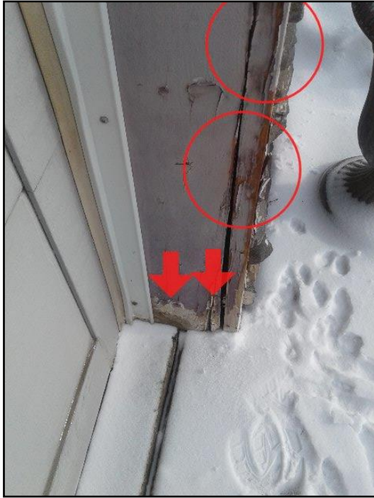
15. Paint or stain needed
