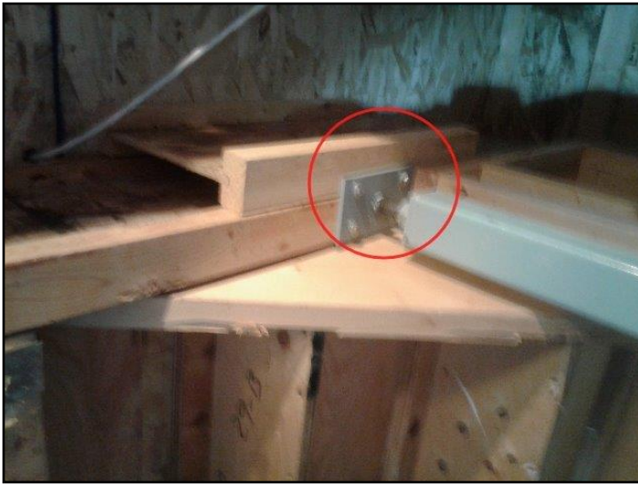
21. Weak connection to joists
