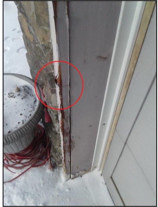
16. Paint or stain needed
